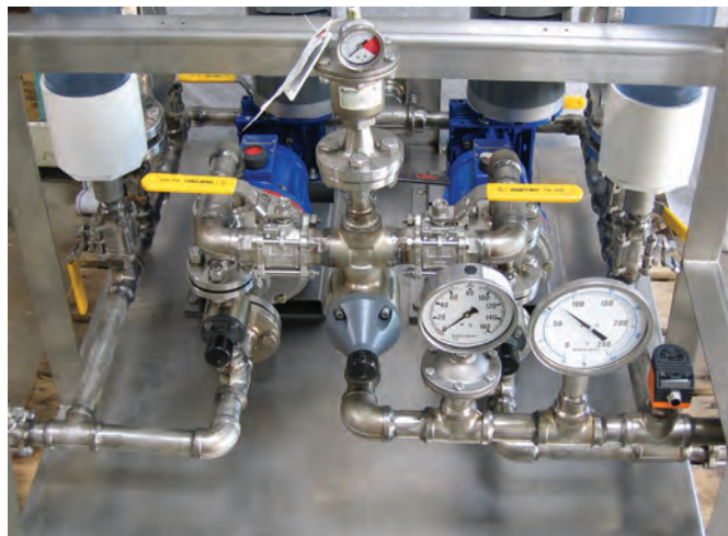
Metering flocculants for wastewater treatment.
