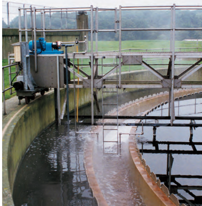
Hydra-Cell operating in a wastewater treatment facility.
